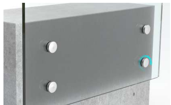
4. Once everything is in place screw on top part of the standoff. Finished look.
